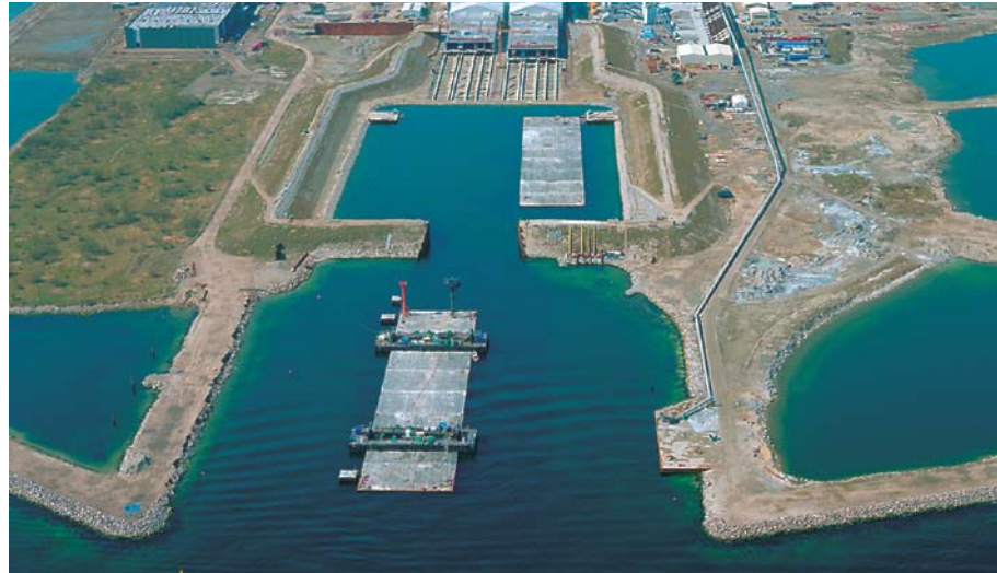
The elements for an immersed tunnel would be cast on land, combined into sections and towed out to the tunnel trench where they would be positioned one by one. Photo of the production facility for the Øresund tunnel.
